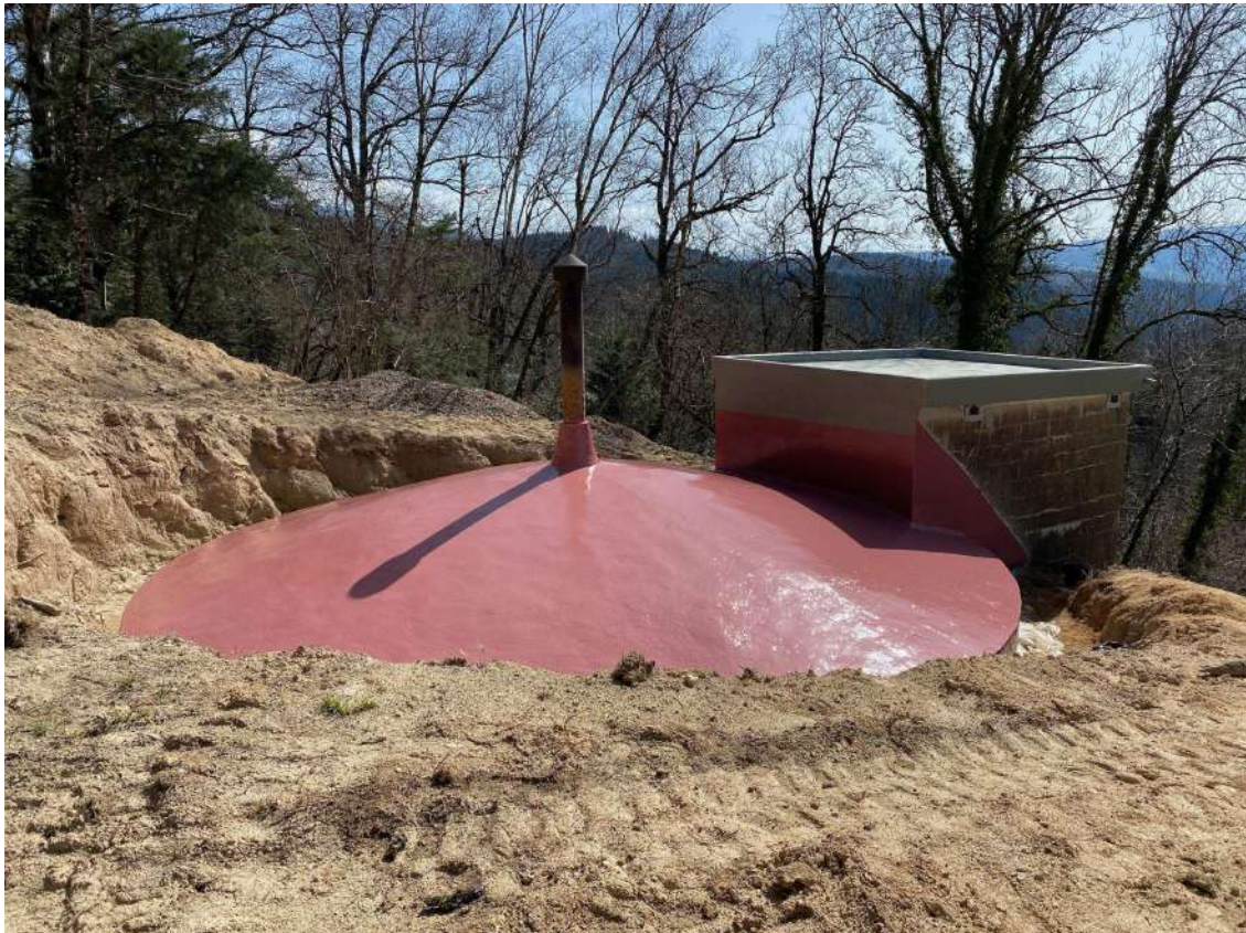
Water tank in Auvergne, March 2020
