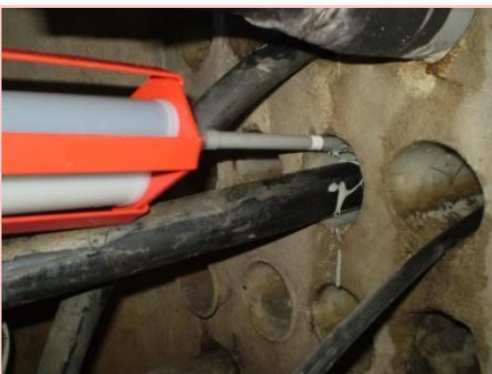
Cables ORANGE injection
